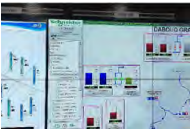
Figure 2-3 Applied SCADA system on all cities and villages in Jordan through WSID
