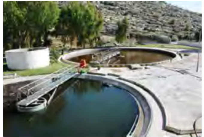
Figure 1-2 Salt City wastewater treatment plant in the middle reaches of Wadi Shueib northwest of Amman City
