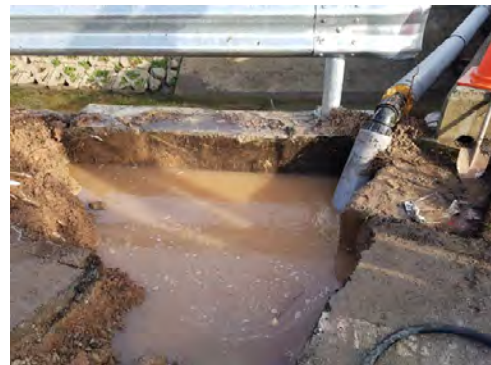
[Leakage in the Bridge Crossing Pipe]
