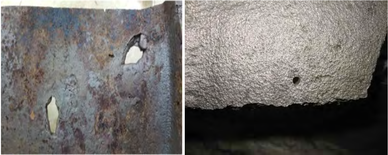
[Internal Hole, Crack, and Burst in Metallic Pipe]
