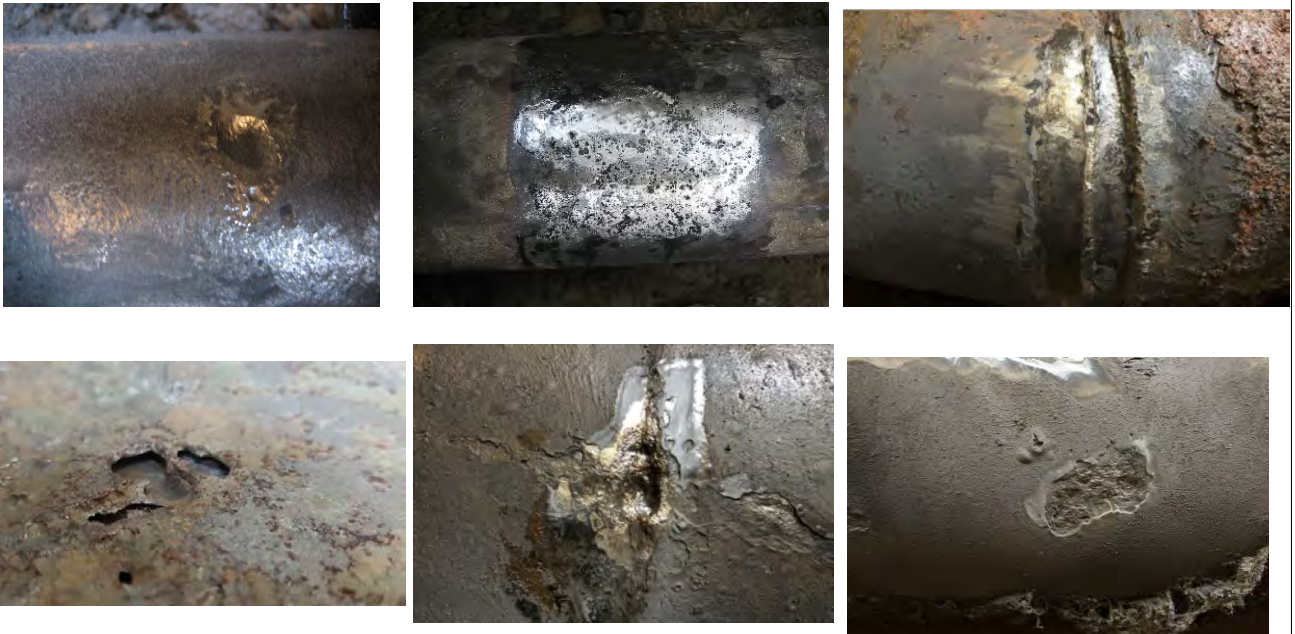
[External Corrosion in Metallic Pipe]
