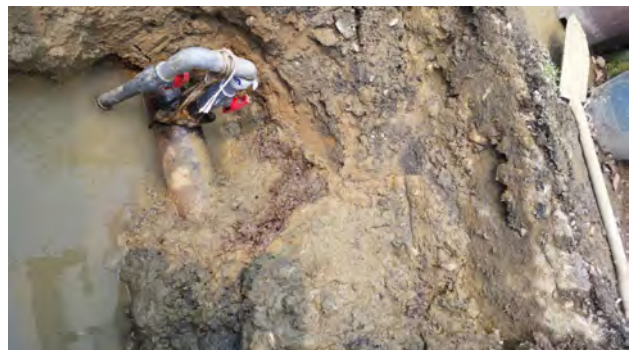
[Improper Repair Using a String or Rubber Band]
