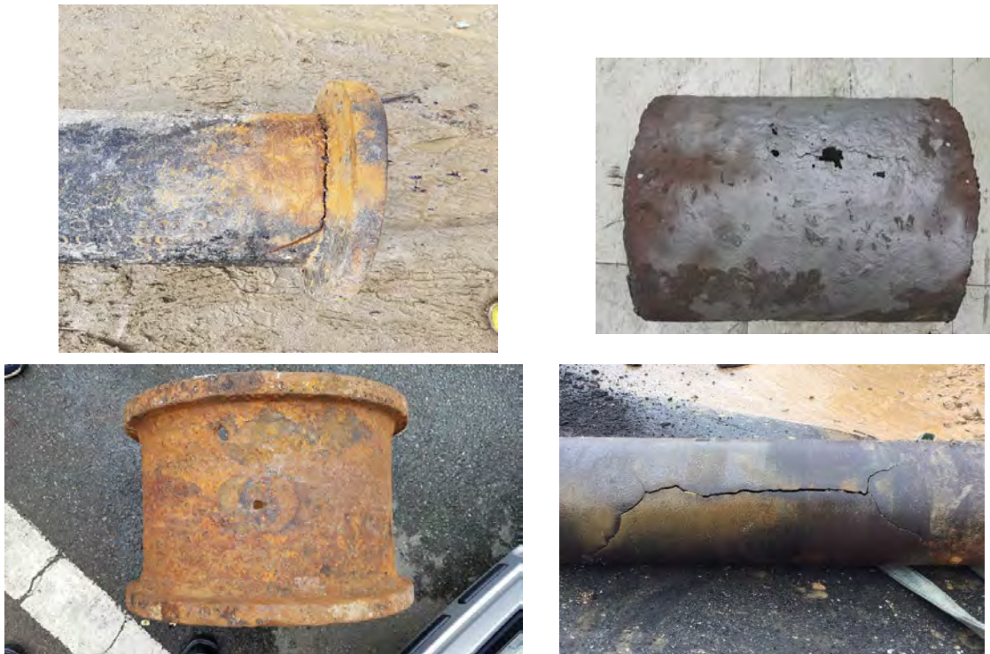
[External Hole, Crack, and Burst in Metallic Pipe]
