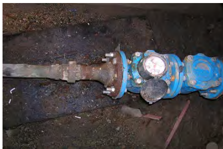
[Improper Meter Size]
