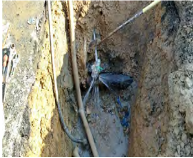
[Leakage at the Saddle]
