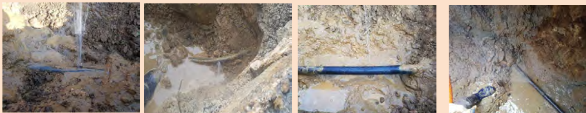
[Reported and Unreported Leakage]
