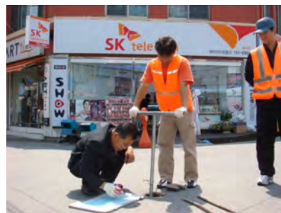
[Preparation for the Test: Step Test Valve Test]
