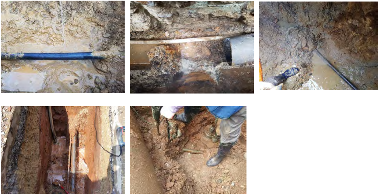
[Leakage in the Aged Pipe #2]
