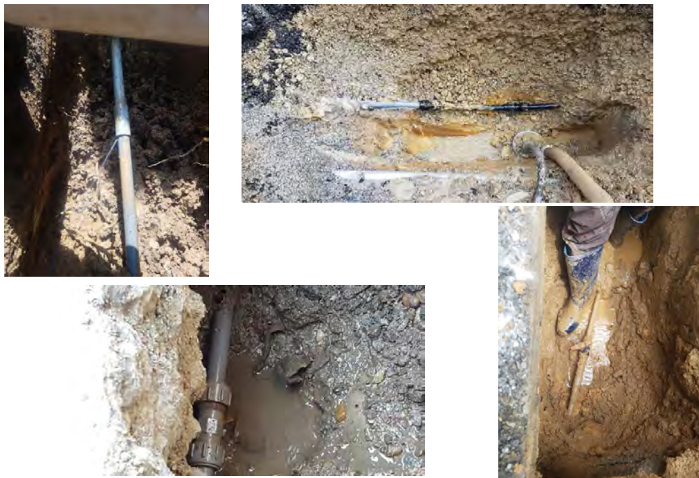
[Leakage in the Aged Joint #2]
