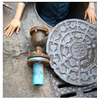
[Leakage at the Air Valve]
