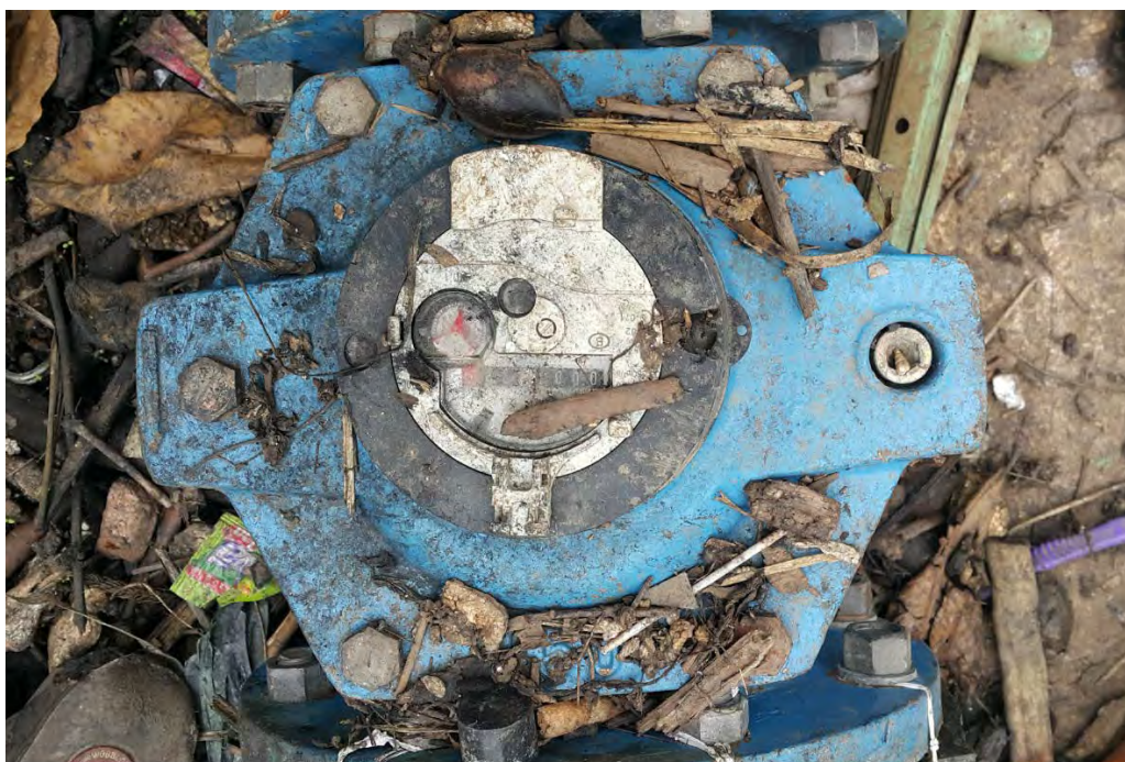
[Stopped Bulk Meter]
