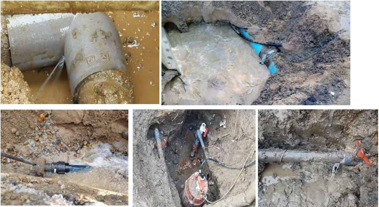
[Leakage in the Aged Joint #1]
