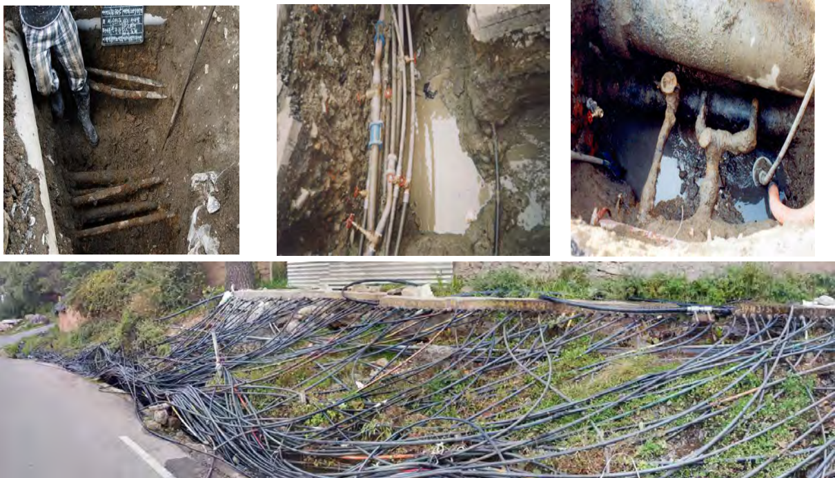
[Leakage in Unorganized Service Connection]
