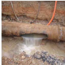
Hole / crack / burst
