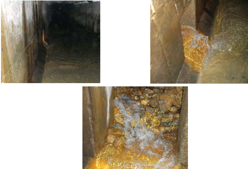
[Analyzing the Result: Leak Location (H Apartment inlet pipe (SP D100 mm) elbow)]
