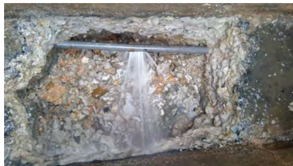
[Leakage Caused by Bad Backfill]
