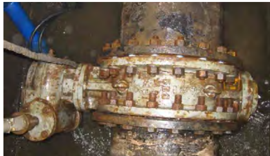
[Leakage at the Aged Valve #2]
