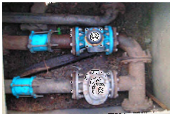
[Improper Meter Installation]
