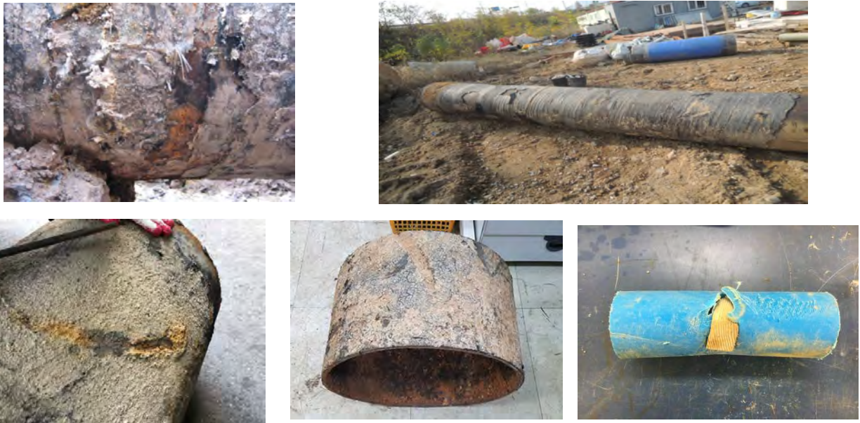
[External Damaged Coating and Taping in Metallic Pipe]
