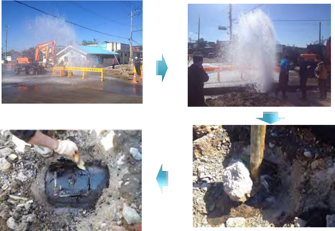
[Pipe Failure and Repair by External Force During Road Construction #2]
