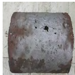
Hole / crack / burst
