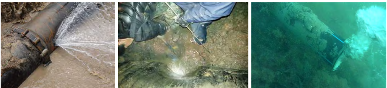
[Leakage from Pipe Broken by External Force]
