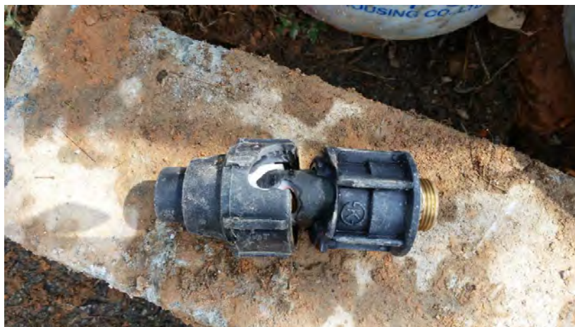
[Damages Caused by High Pressure]
