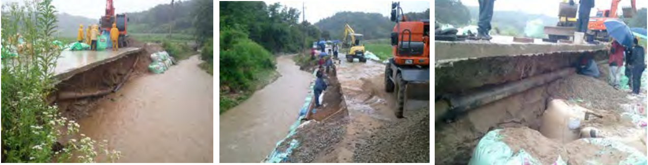
[Loss and Restoration of Pipelines due to Heavy Rain]
