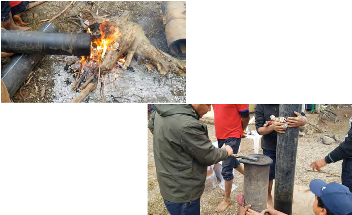
[Improper Joint Connection]
