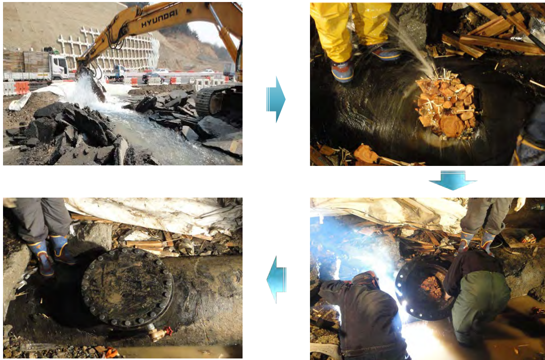
[Pipe Failure and Repair by External Force During Road Construction #1]
