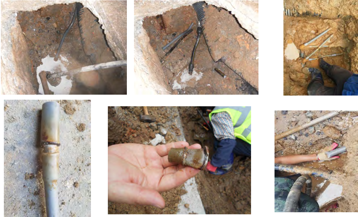
[Leakage at the Unproperly Deformed Pipe using Heat in the Field]
