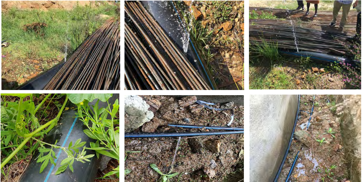
[Leakage in Exposed pipe]
