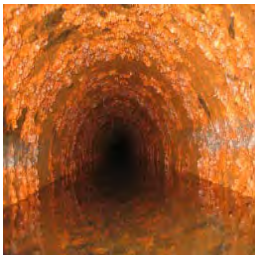
Local internal corrosion
