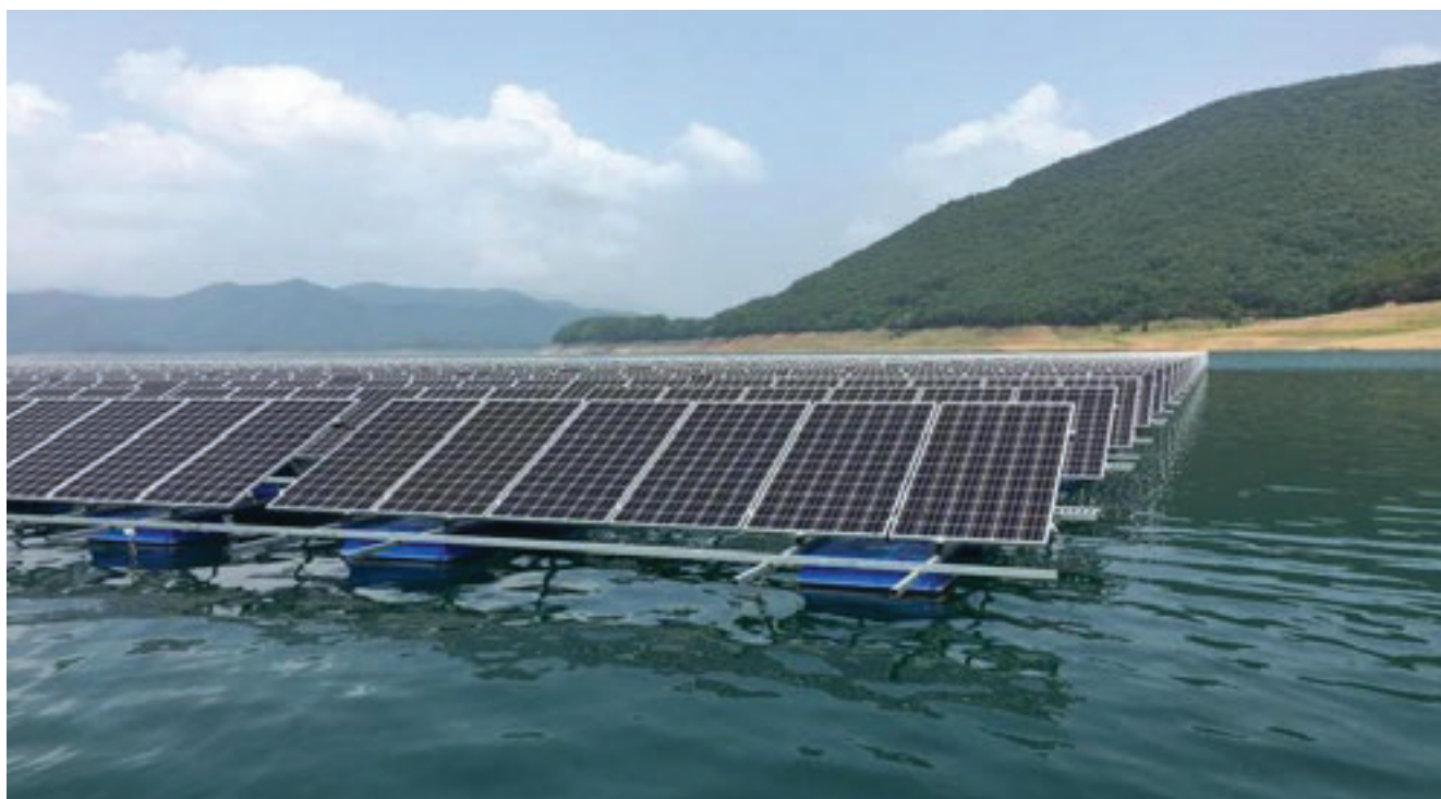
Figure 9-8 Floating solar power plant on the surface of the reservoir at Chungju Dam (Source Jecheon City Hall, January 2018)
